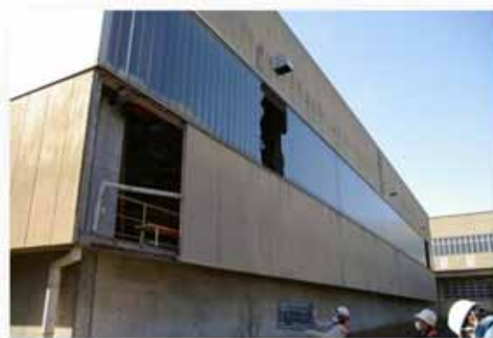
Damages to the General Gymnasium
