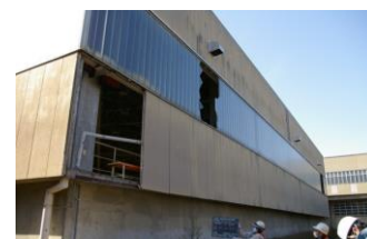
Damages to Multi-purpose Gymnasium (at the time of the earthquake)
